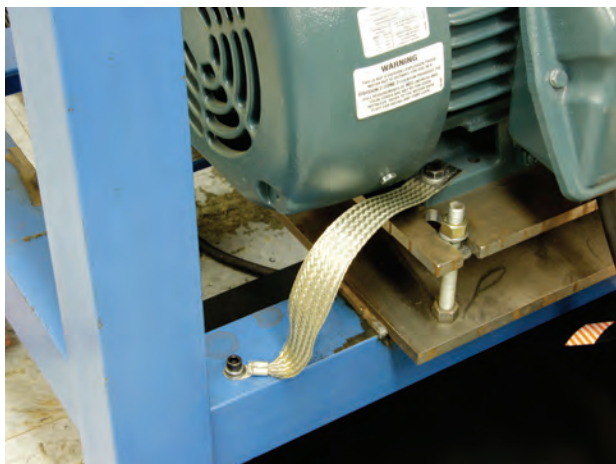
Motor frame bonded to its support by a high frequency grounding strap
